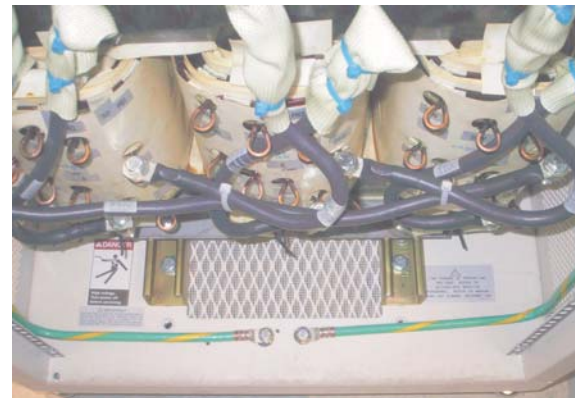
A view of the inside of a typical TEAL power subsystem containing a 3-phase isolation transformer. The transformer taps for various input voltages are easily accessible "loops" and can be switched in a matter of minutes.
